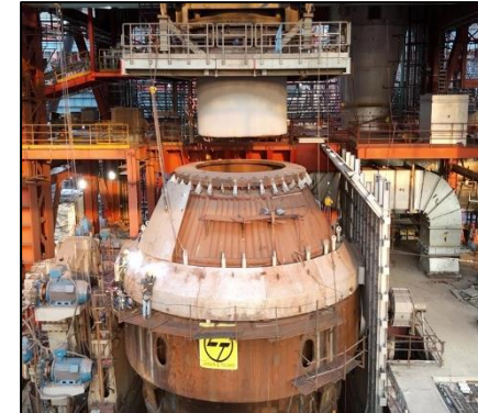
Converter-2 at SMS
